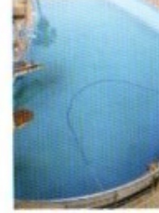
Pipeless Filter in Big Pool at SURAT
